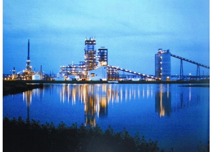
Utility companies are pursuing IGCC projects in preparation for carbon emission restrictions which will come. (IGCC plant at Mulberry, FL pictured above)
