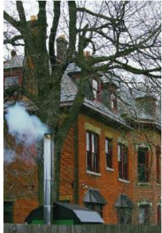
A wood-fired boiler in Columbus, Ohio 1
